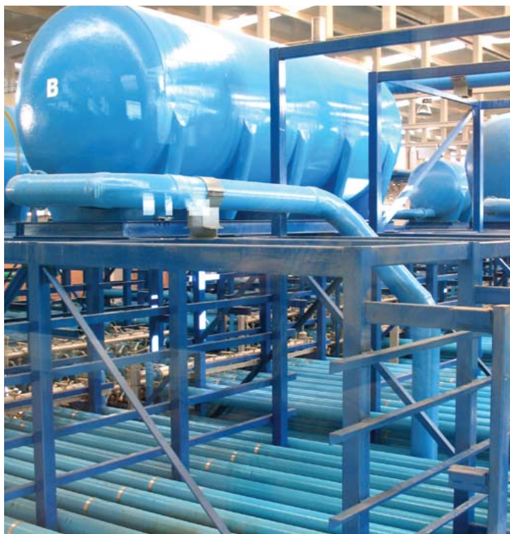
High-pressure pumps push sea water through reverse osmosis membranes housed in narrow blue tubes. Above, desalinated water is stored in tanks to flush seawater at shutdown.
